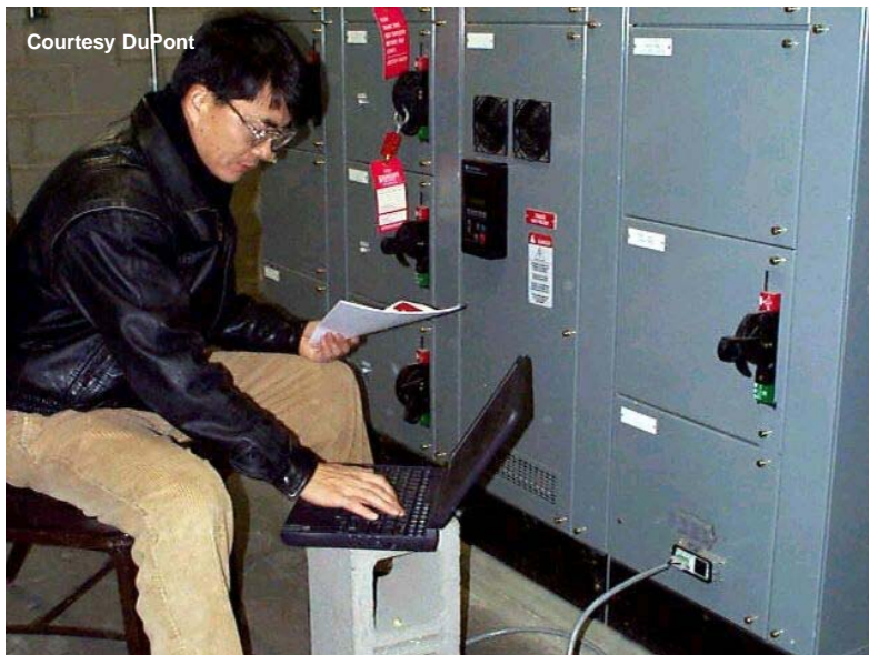
Smart MCC troubleshooting
