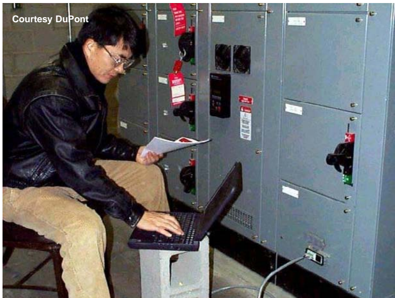
Smart MCC troubleshooting
