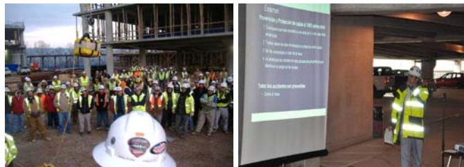
Workers have the right to know what a safe workplace looks like and what hazards they face.
