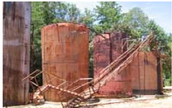
Damaged oil tanks involved in the June 5, 2006 explosion and fire at Partridge-Raleigh Oilfield.
