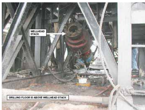
Wellhead stack involved in the incident.
